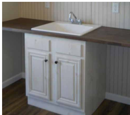
Laundry Sink with Cabinets
